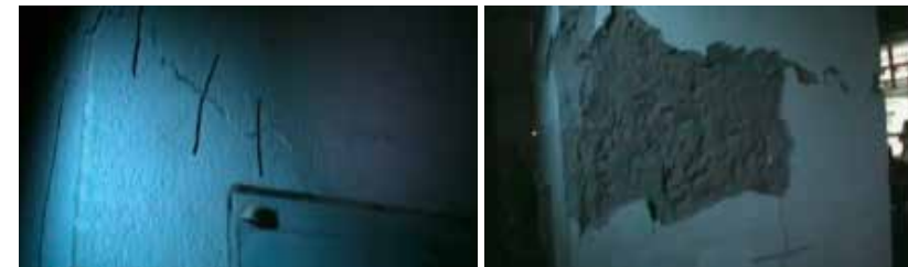
Figs. 3, 4. Stills from a Dhaka police video showing building surveyors' markings over the crack (image on the left) in one of Rana Plaza's walls, Savar, Dhaka area, April 23, 2013 (a day before the collapse). Source: "Dhaka Building Collapse: Police footage shows cracks," BBC News, April 26, 2013 http://www.bbc.co.uk/news/world-asia-22307589 .
